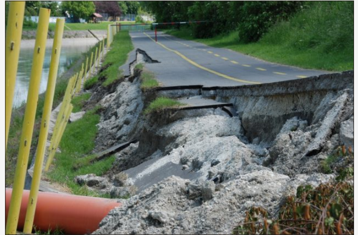
Fig.2 Damage on the bicycle road between Siófok and Siójut caused by heavy precipitation and landslide (Photo: Ákos Horváth).
